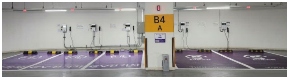
Five slow chargers (AC) at headquarters
